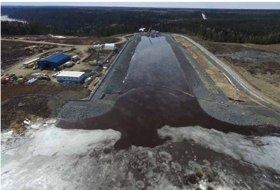
The completed intake channel on the upper portion of the New Post Creek.
