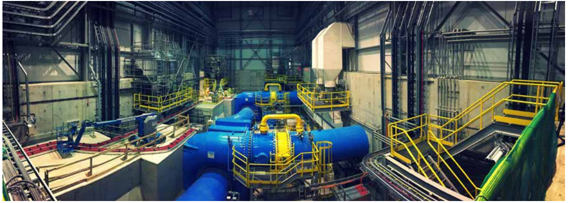
A photo inside the powerhouse showing the two horizontal axis Francis turbines in place.
