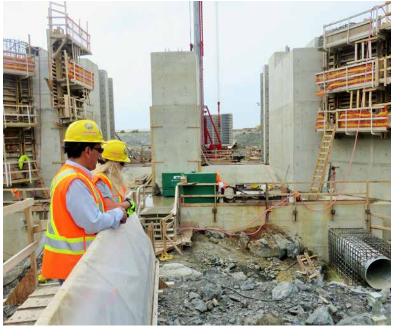
President Wayne Ross and First Nations Project Manager Sue Hartwig at the powerhouse construction site.
